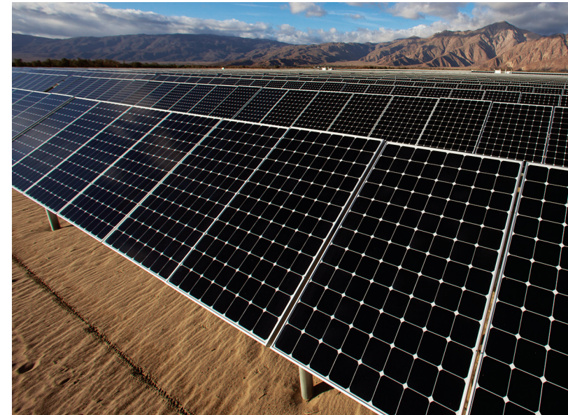
Borrego Solar Generating Station, CA
